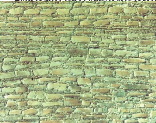
Plate 4.7. Time and space in one document. A wall from Chaco Canyon with two construction styles evident, New Mexico, USA (Photograph: R.R. Dods 1991).
