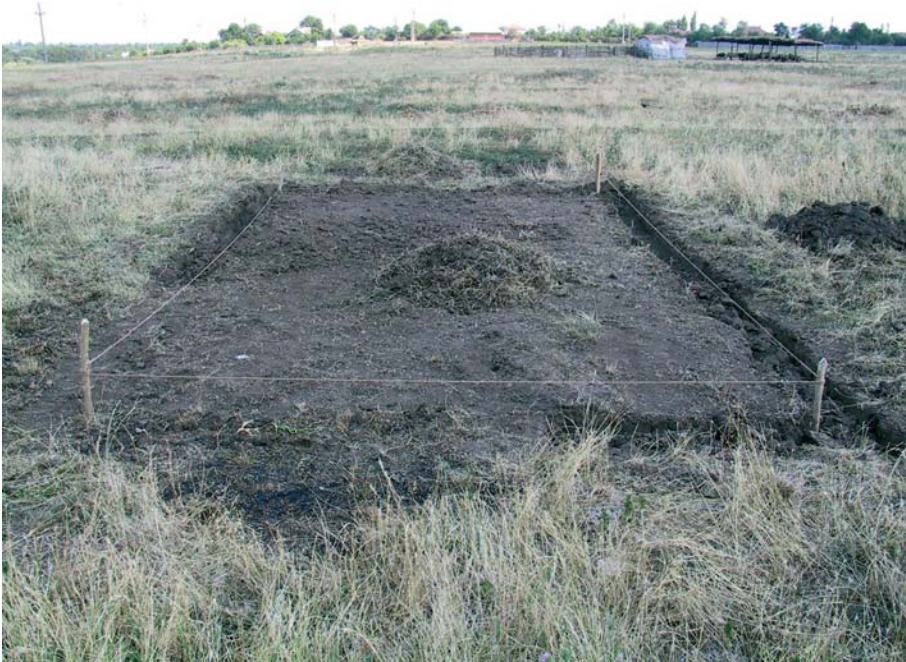
Figure 12.10. The fiber frame for tracing the foundation trench of a wattle and daub house.
